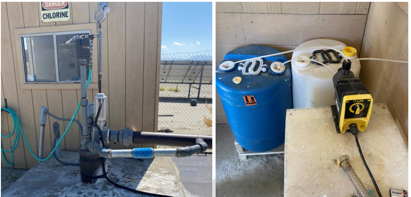
Figure 3 Image at left shows the groundwater well and the submersible pump connections for the KCSD Water System. Image at right shows the chlorination treatment of the groundwater at the well site prior to entering the distribution system.
