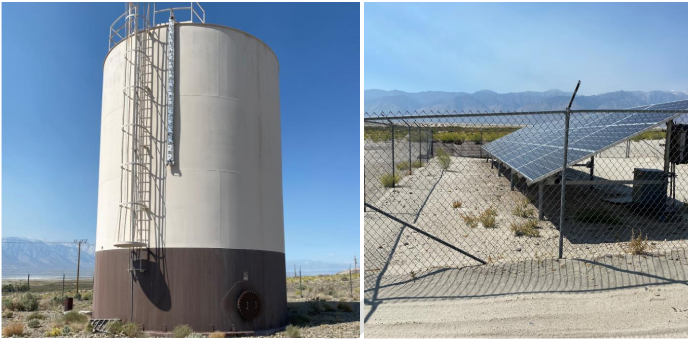
Figure 4 Image at left shows the 100,000-gallon storage tank. Image at right presents the solar equipment used to power the pump system at the groundwater well.
